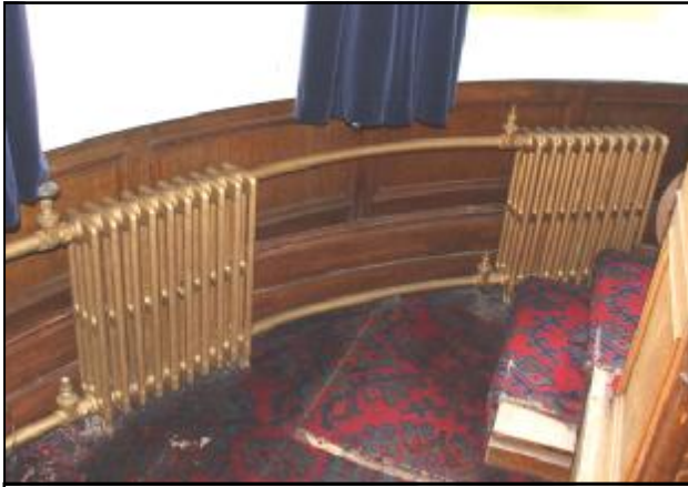
Radiators to curved wall
