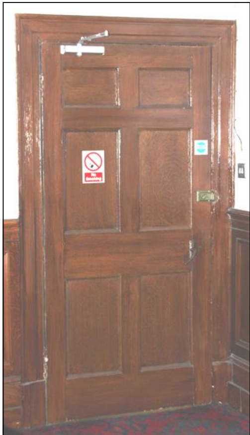
Entrance door with original paneling and architraves but all original door furniture has been removed.
